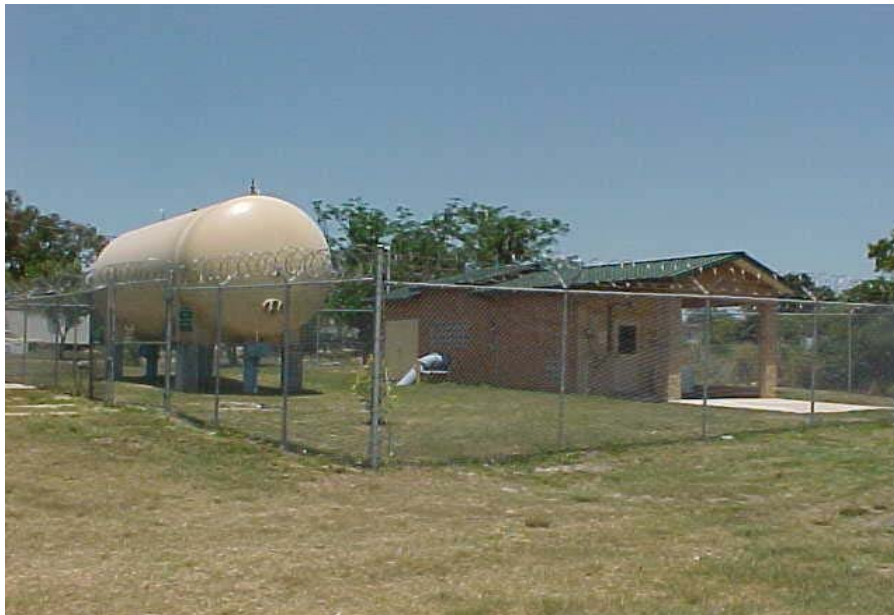
# 2 SIRENA WATER TREATMENT PLANT
